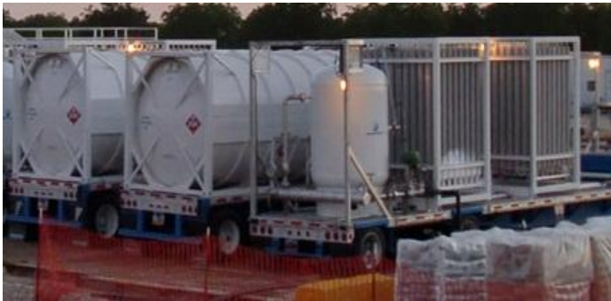
PHOTO COURTESY OF PROMETHEUS ENERGY
